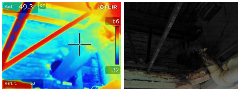
Cold spots indicated by the blue color. There are several holes that penetrate the wall and go through the space above the parking spots
